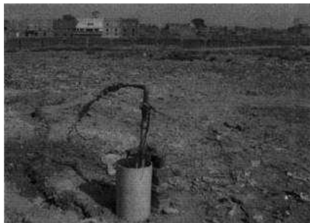
Step vi: Drawing water samples by installation of submersible pump in constructed well
